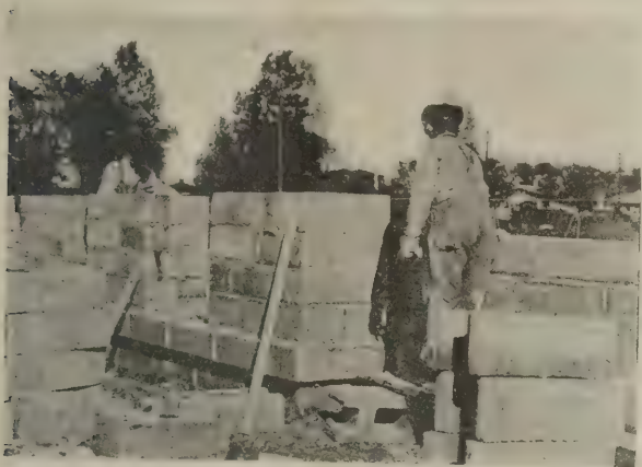
When stone masons are not available, training will help brick masons increase their capacity for laying concrete block
